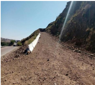
EAR at the 253rd km of Angren-Pop route. The slope of the road at the location of EAR is 12%;
