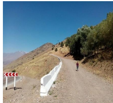
Pop-Angren route EAR at 222 km. The slope of the road at the location of EAR is 12%;
