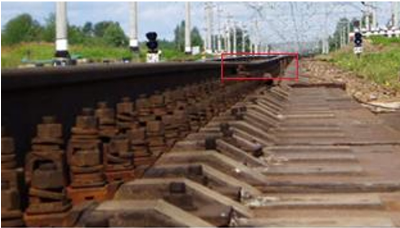
Fig. 1. Deformations of the embankment at the interface with the bridge [5]
