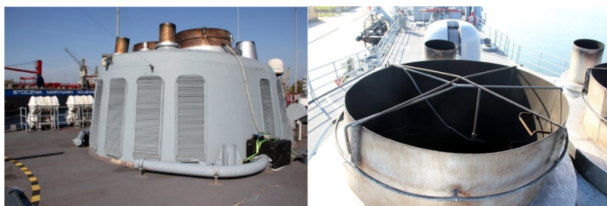
Fig. 4. Superstructure on the upper deck with the exhaust system and view of the probe mounted in the exhaust outlet.
