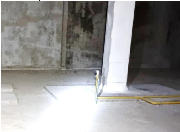
Fig. 2. Erroneous reinforcement of the support zone of the column from above is an incorrect definition of the problem
