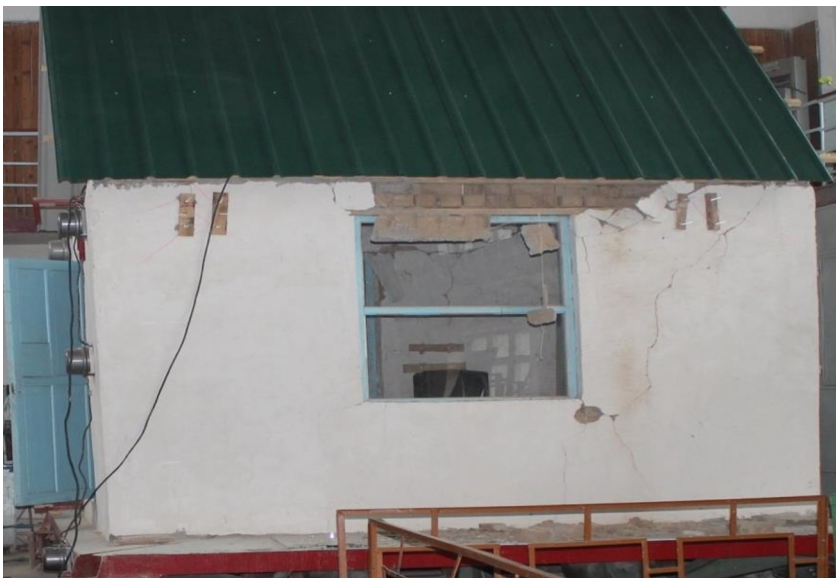
Fig. 2. General view of the model of the house, made of brick raw, after the experiment
