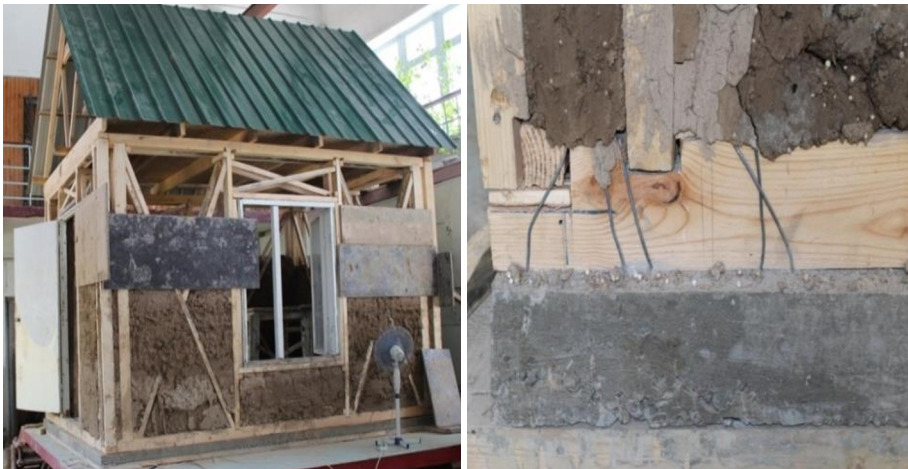
Fig. 3. The process of construction of a model house of wooden frame "synch".
