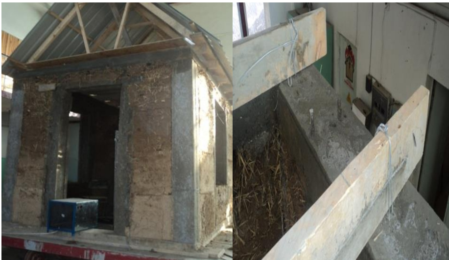
Fig. 5. The process of construction of model homes from the «reinforced concrete frame».
