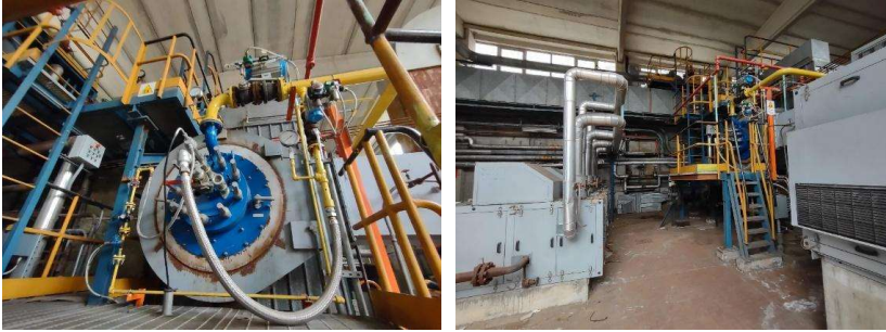
Figure 1 – The water-tube boiler of the Tirreno Power combined cycle plant of Quiliano (SV), Italy; front view (on the left) and side view including the water pumps (on the right).
