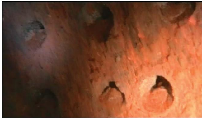
Fig. 2. Clogged filter porous by salt sediments and corrosion products (Photo by Abror Gadaev during the CCTV inspection of the water well).
