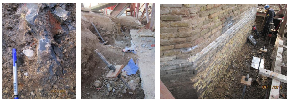
Figure 14: Views of the vertical and inclined micropiles implemented near the seat of the Minaret of Dhu Al-Kifil Nabi (PBUH) along with the size of the injected area.
