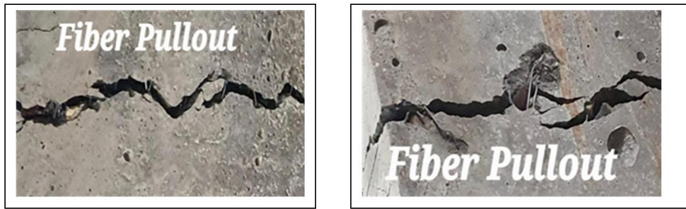
(a) Crack of a prism with micro steel fiber.
