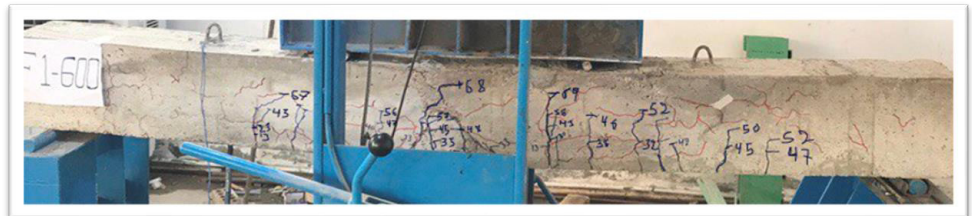
Figure 17: Cracks pattern for the specimen (F1-600).
