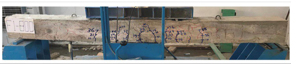
Figure 19: Cracks pattern for the specimen (F1-800).
