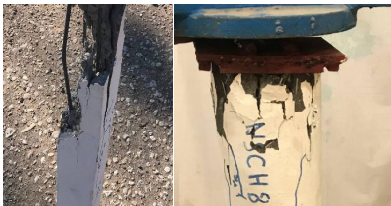
Figure 11: Failure Pattern of (left) NSC column strengthened with SIFCON shell, (right) NSC column.
