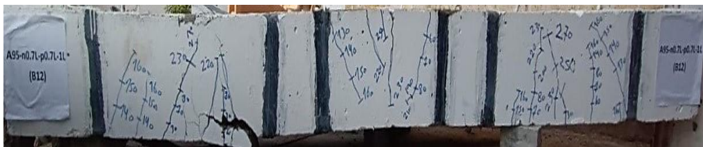
Figure 12: Map of cracks for A95-p0.7L-n0.7L-1L.
