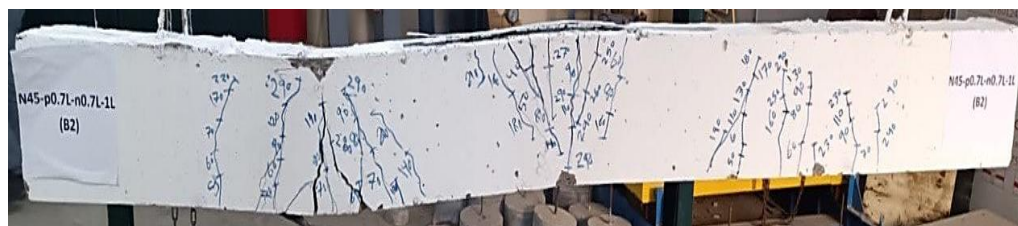
Figure 6: Map of cracks for N45-p0.7L-n0.7L-1L
