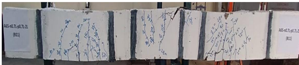
Figure 11: Map of cracks for A65-p0.7L-n0.7L-2L.
