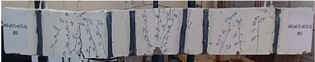
Figure 7: Map of cracks for A45-p0.7L-n0.7L-1L.
