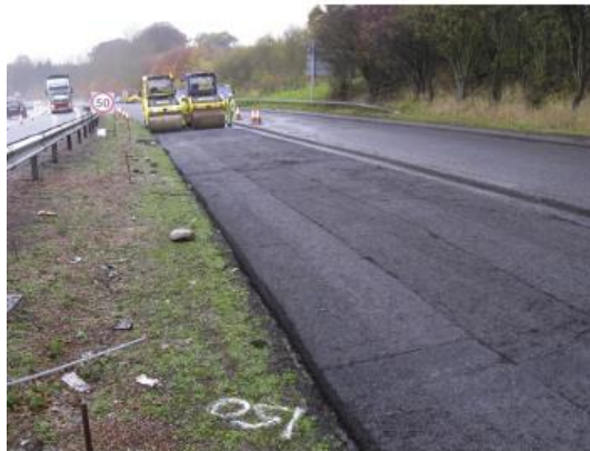
Figure 6: Application of cold mix asphalt on A90 trunk road site before compaction [71].
