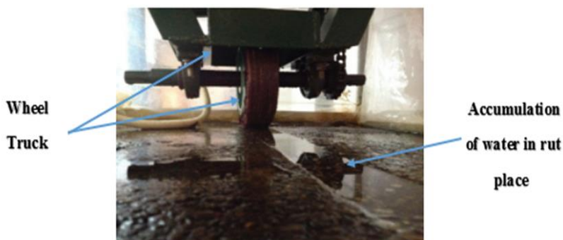
Figure 12: Resulting rutting on the pavement.
