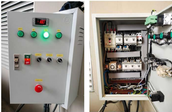
Fig. 5. The refrigeration system control box.
