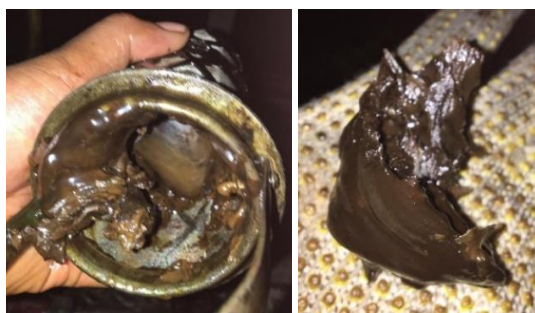
Fig. 3. Blockage in the strainer booster module.
