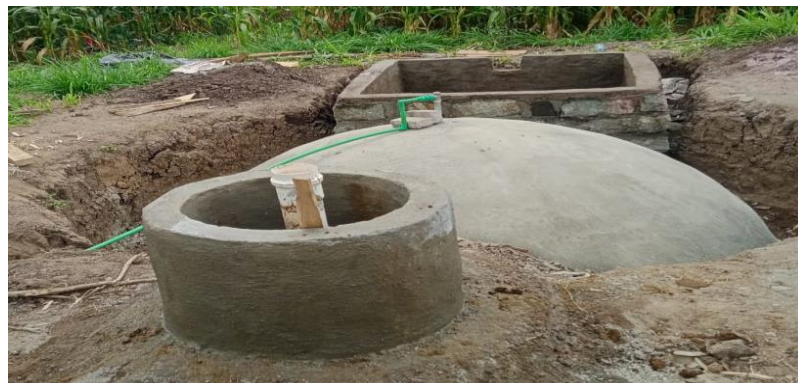
Fig. 4. Fixed Dome Digester
