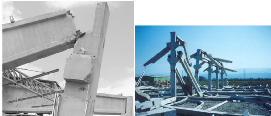
Fig. 1. Structural failures of precast elements in beam-column connections in building structures due to seismic loads [4]
