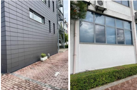
Fig. 2. A. Masonry wall with ventilated facade; B. Masonry wall without ventilated facade. (Source: Authors).
