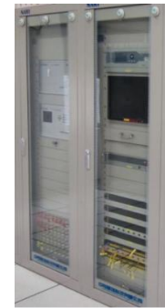
Fig.6 Photo of control & protection system cabinet of SVG
