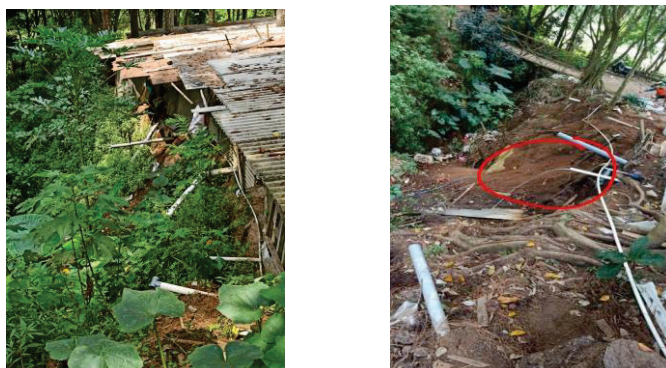
Fig. 1. The existing condition of wastewater discharging at BSC
