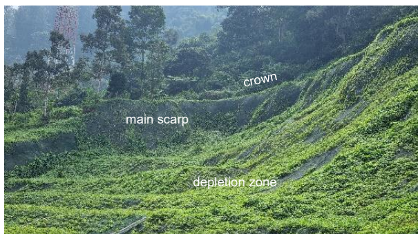
Fig. 4. Cugenang landslide showing the distinct horseshoe-shaped of the crown and main scarp and the depletion zone.
