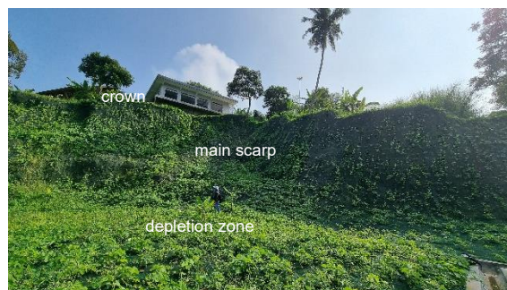
Fig. 3. Cijedil landslide showing the crown, main scarp and depletion zone.
